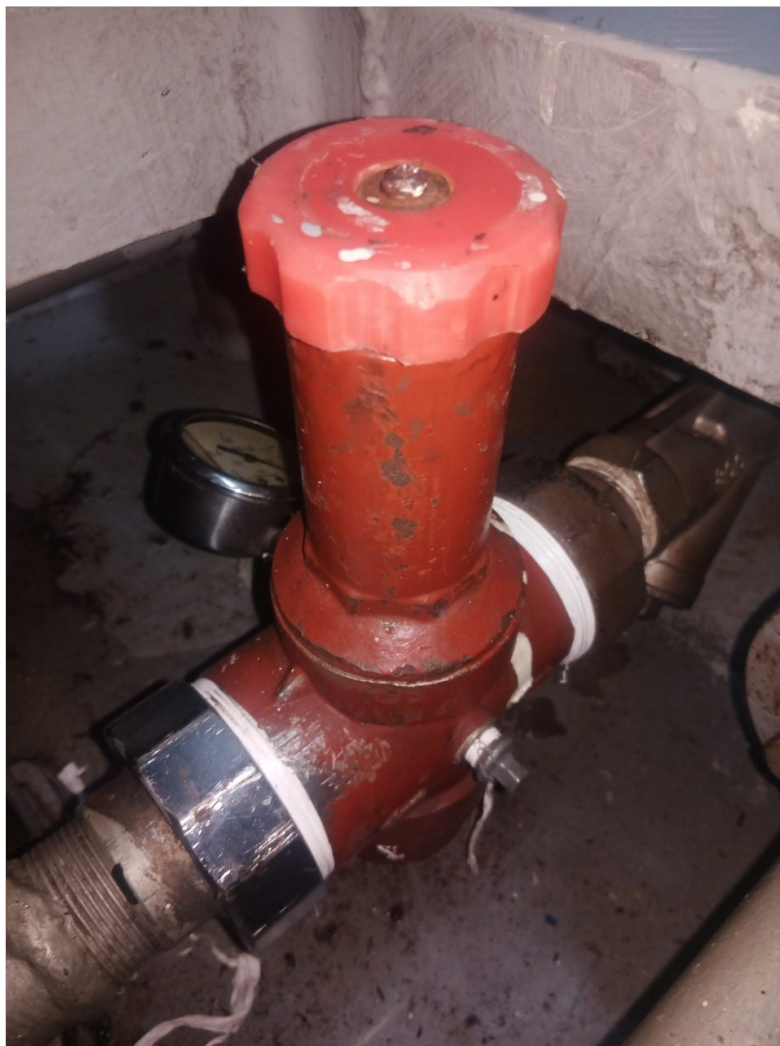
Valvula de control defectuosa
